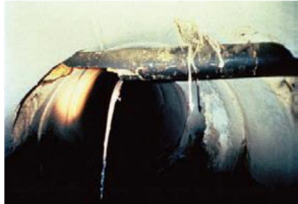
Sewer Pipe Discharging to Storm Drain
