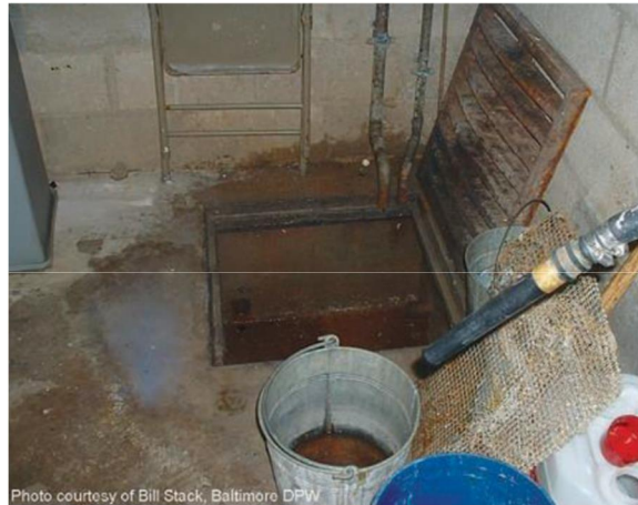
Cross-Connected Floor Drain
