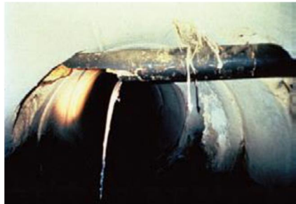
Sewer Pipe Discharging to Storm Drain
